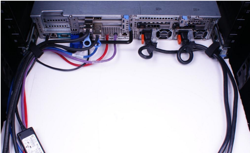
Figure 11. Cabling a system installed in static rails
